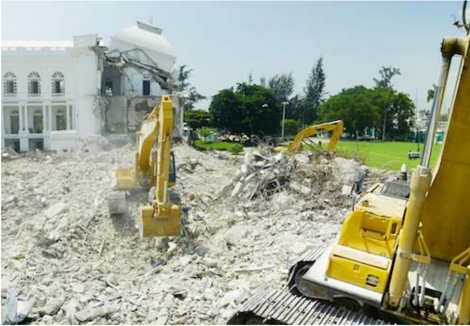
Above: demolition work on Haiti's national palace (Photo: J/P Haitian Relief Organization)
